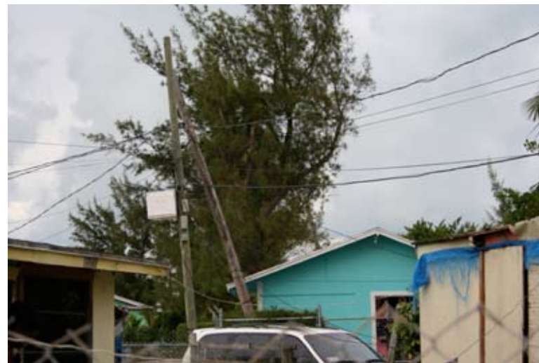
UNSAFE ELECTRICAL WIRING
