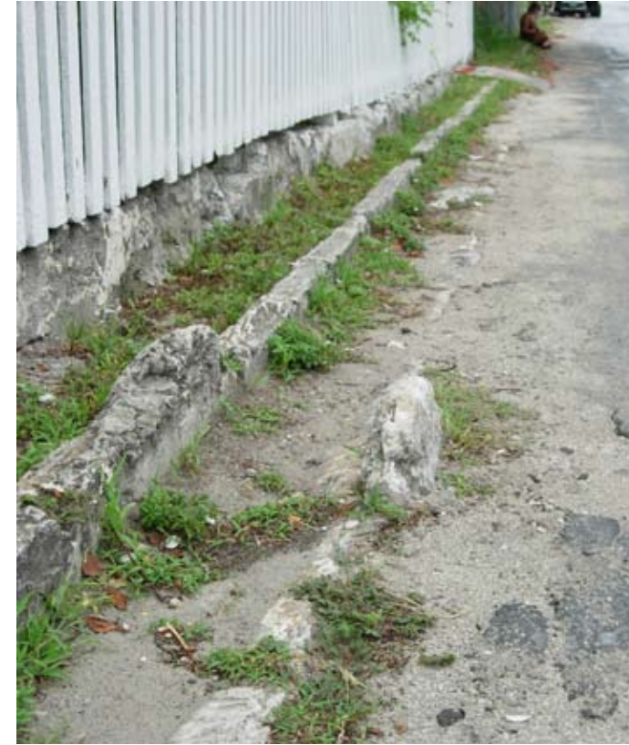
T4: Open Gutter, Dunmore Street
