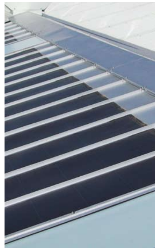
ROOF INTEGRATED SOLAR PANELS
