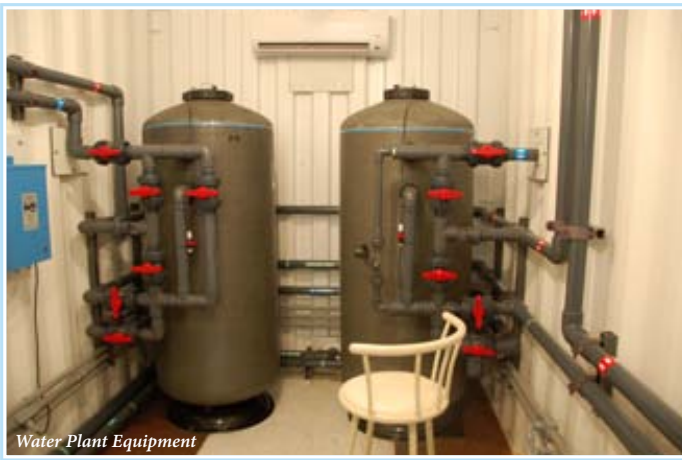
Water Plant Equipment
